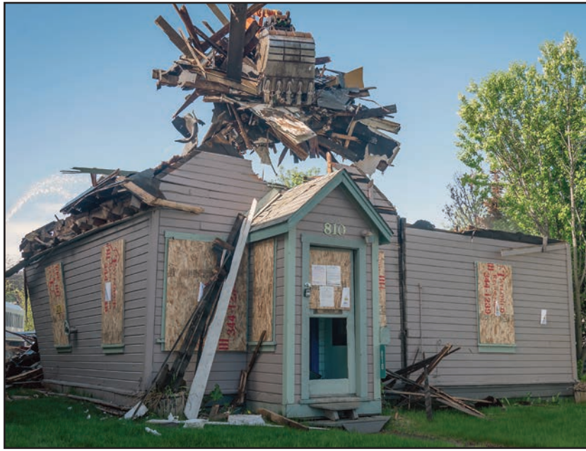
A demolition crew takes down the Amundsen House in downtown Anchorage on May 30, 2024.
